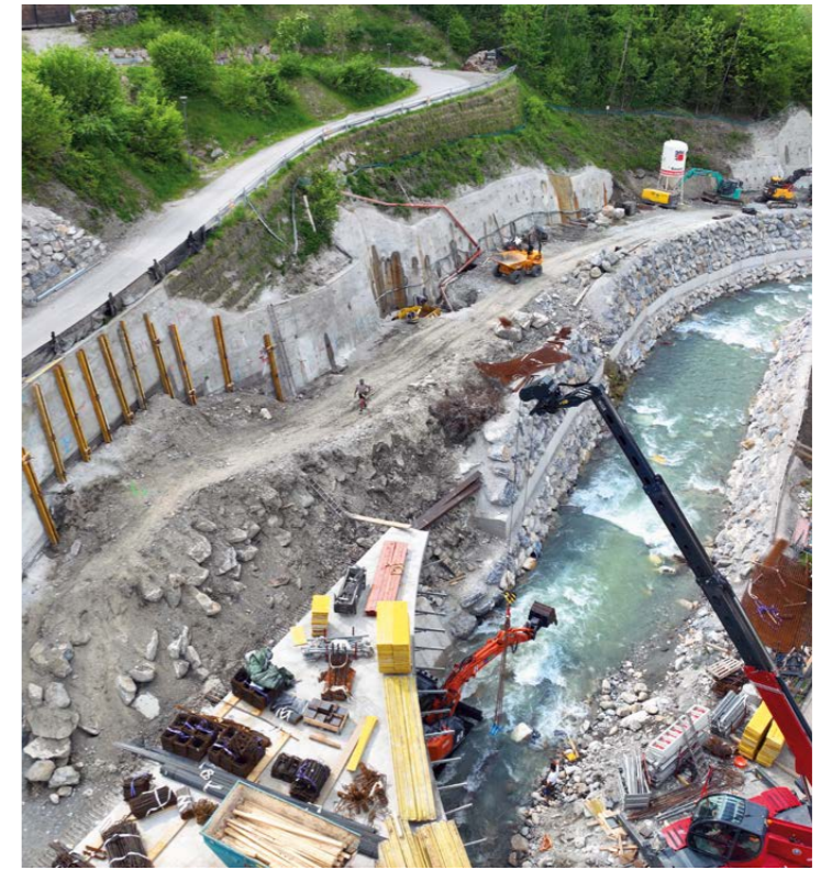
Hydroelectric Power Plant, Wagrain, Austria
