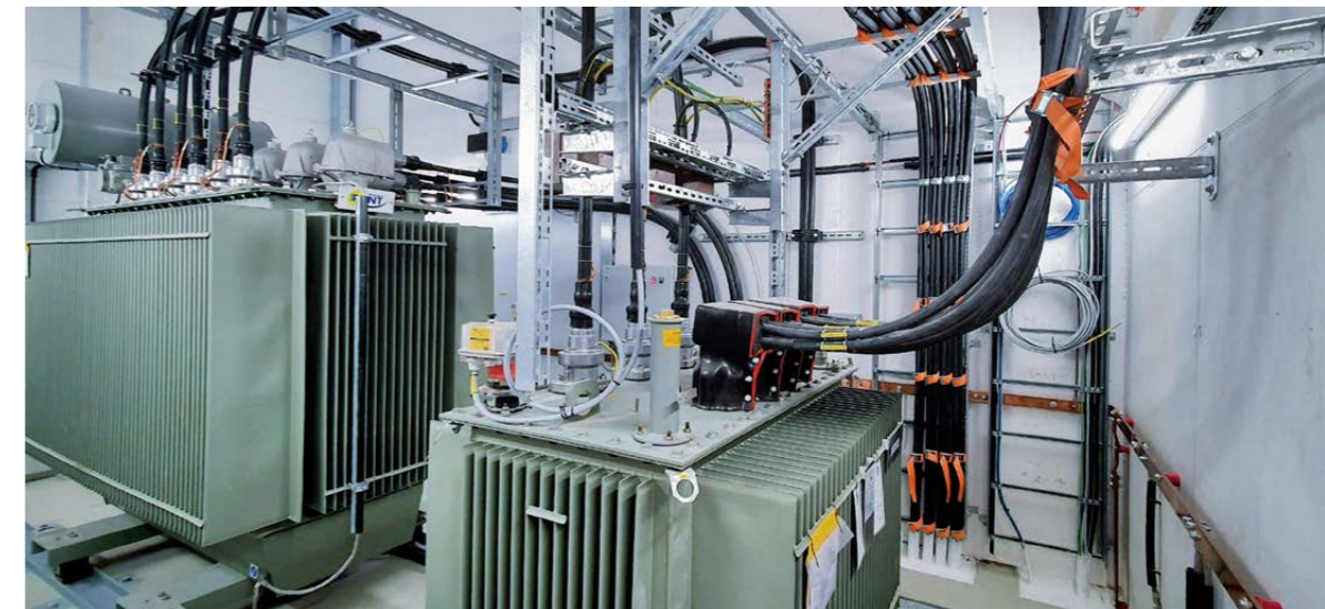
Electrical Installation, Töging Power Plant, Germany
